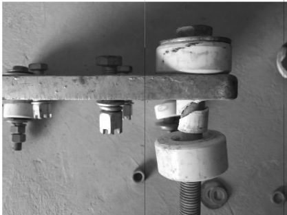
图 3 2029 号避雷器绝缘底座瓷套破损情况 Fig. 3 No. 2029 insulation base damaged conditions
